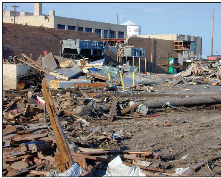
The Hoisington tornado damaged the high school, a small shopping center, the hospital and hundreds of homes in a matter of minutes. (photo by Dave Saville/FEMA News)
