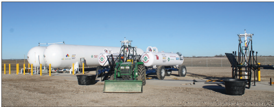
MKC improvements made recently include a new anhydrous facility. The facility includes two anhydrous tanks which hold a combined total of 56,000 gallons of anhydrous along with four filling stations.
