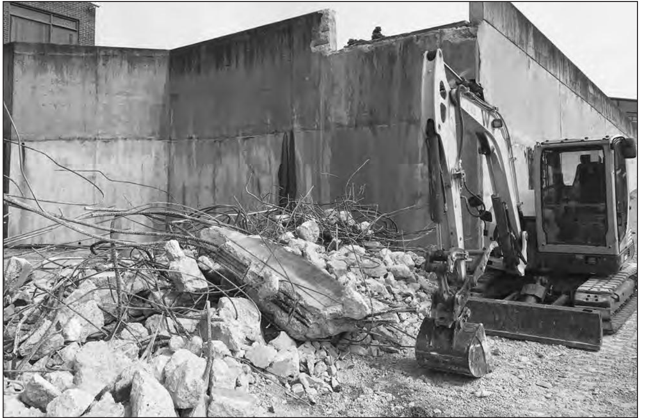
Warren County Middle School has lost one of its concrete walkways. The bridge was reduced to rubble by Midwest Maintenance without incident, which could pave the way for the company to receive payment on prior, but unauthorized, work.
