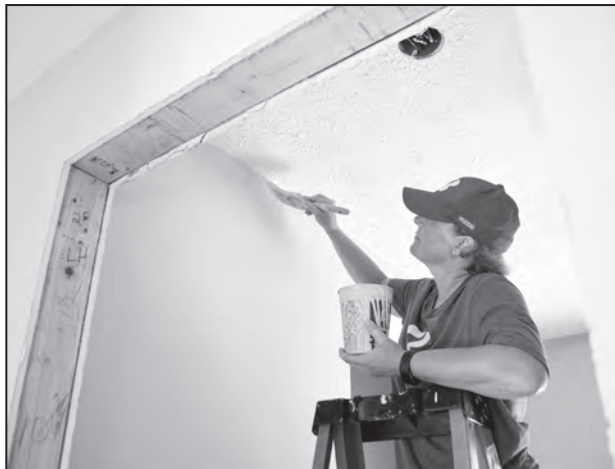
Lacy Garrison photo Bridgestone plant manager Tamara Martensen uses a paint brush to do edging in the front bedroom of the 31st Habitat home on Tuesday. "There is a lot of sweat and work that goes into it from a volunteer's perspective, but it is one of the most rewarding things that I think you can do ... to actually know you're creating a structure for a family," said Martensen.
