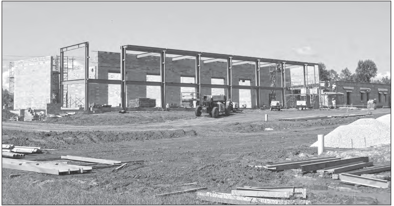
The Automation & Robotics Training Center is under construction in McMinnville and is scheduled to offer non-credit classes in May 2019.
