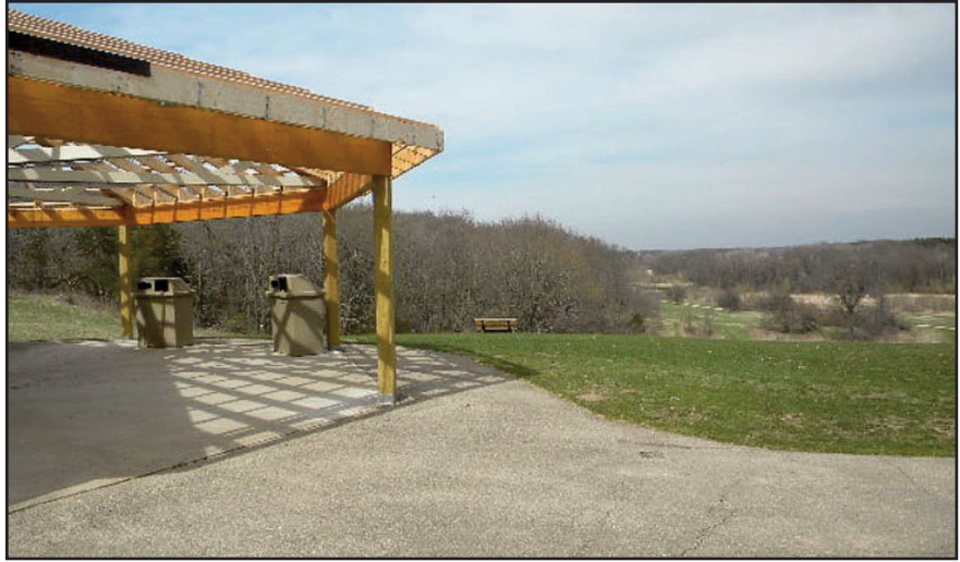
Shelter #3 in Cam-Rock Park is undergoing a rebuild. (Photos by Janice Redford)
