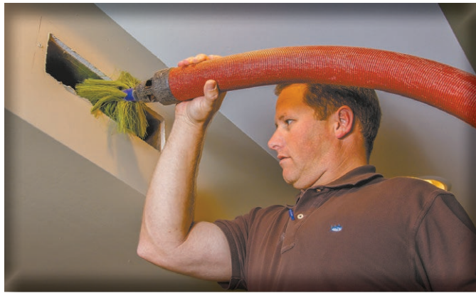
Ducts may need to be serviced by professionals in homes where indoor air quality is poor.
