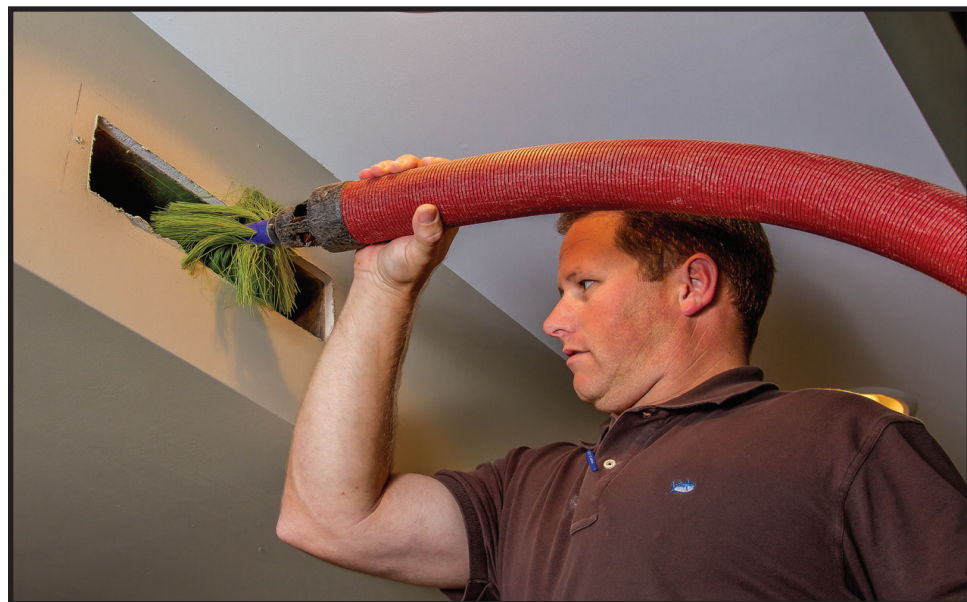
Ducts may need to be serviced by professionals in homes where indoor air quality is poor.
