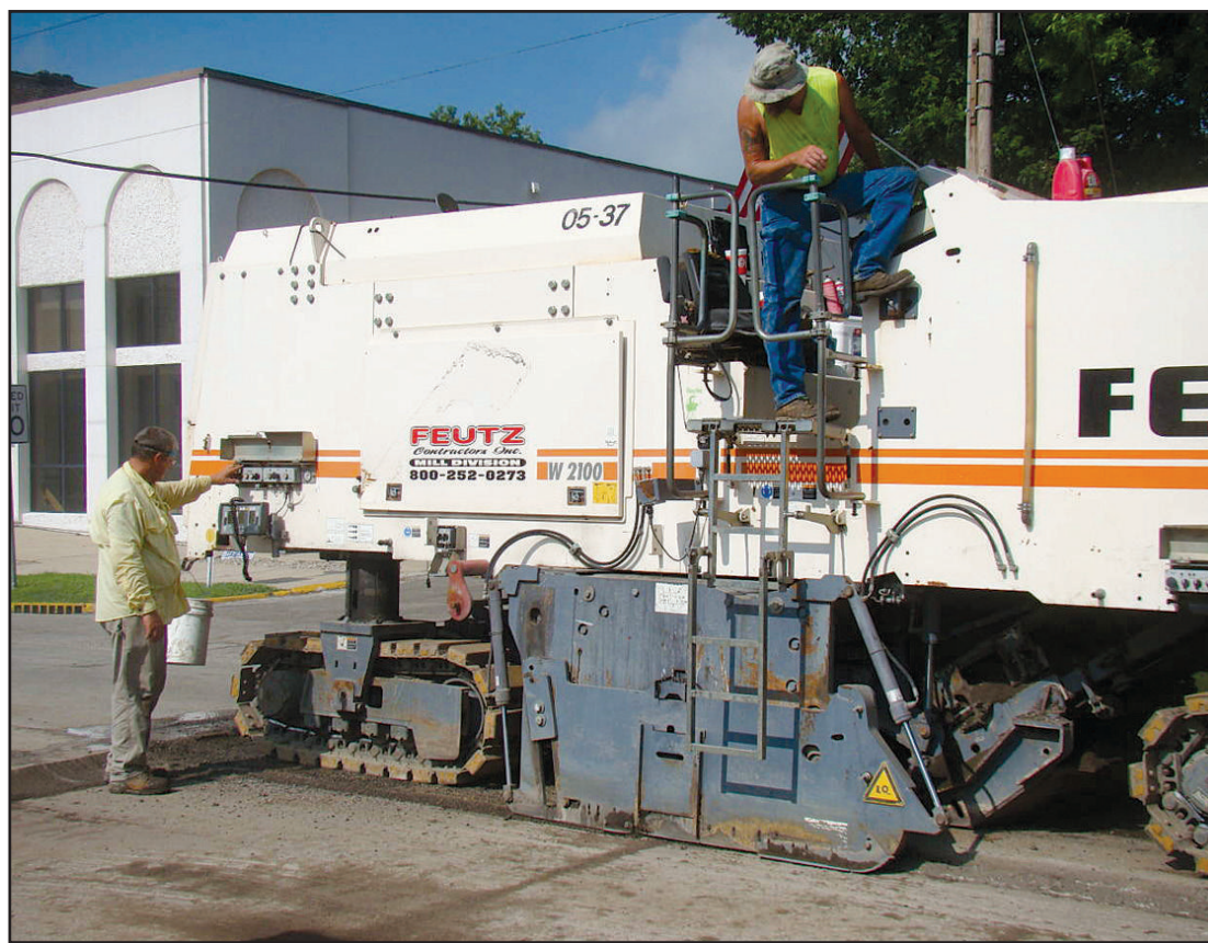
The man on the ground is setting the depth of how much asphalt to grind away.
