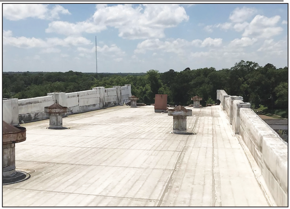
The west end roof of the former Masonic Lodge building, currently owned by Holmes County, on the Lexington Court Square, suffered damage and subsequently collapsed. The damaged went through to the first floor where the Holmes County Chamber of Commerce office was housed. The chamber is currently seeking a new location. The photo was taken on May 22. (Photo by Landon Voller/Belinda Stewart Architects)
