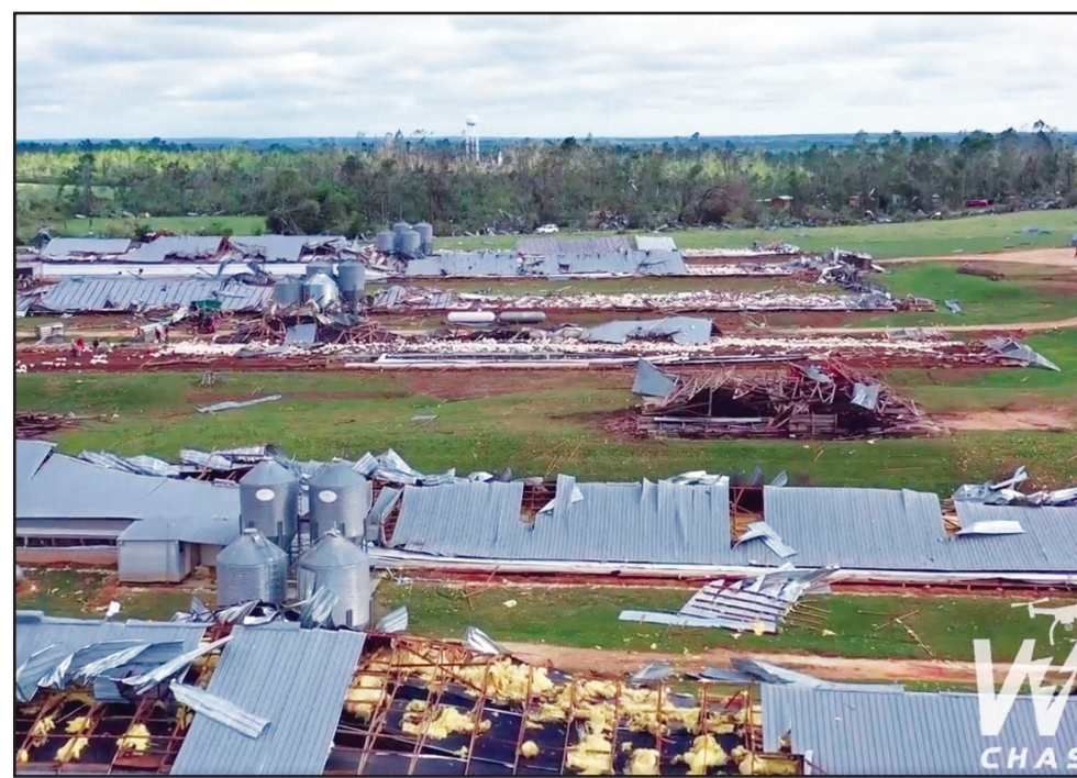
Mississippi's poultry industry sustained heavy losses from storms that ripped through the state Easter afternoon and evening. These poultry houses near Soso in Jones County, Mississippi, were destroyed by tornado April 12, 2020. (Photo by WXChasing)
