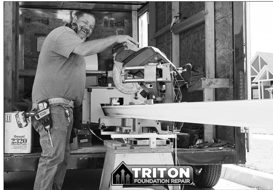
A Triton Foundation repair employee operates an articulating radial arm saw during a construction project. Triton Foundation Repair, owned and operated by Jeff Wedig, is located at 115 Snow Drive in Newcastle, and offers a long list of services. For information about what Triton Foundation can do for you, if necessary, call (405) 437-9031.
