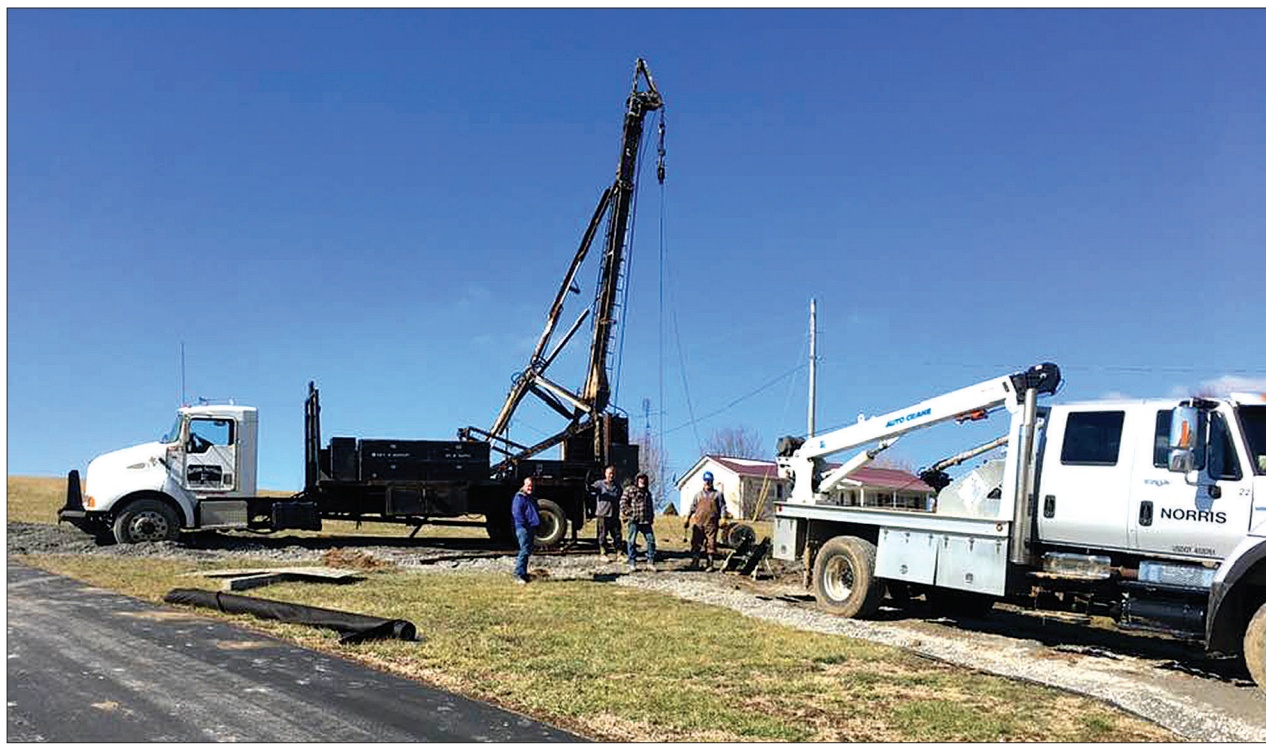
Workers prepare the rig for drilling on property owned by Connie Stotts. Photo courtesy of Vicky Browning Pike
