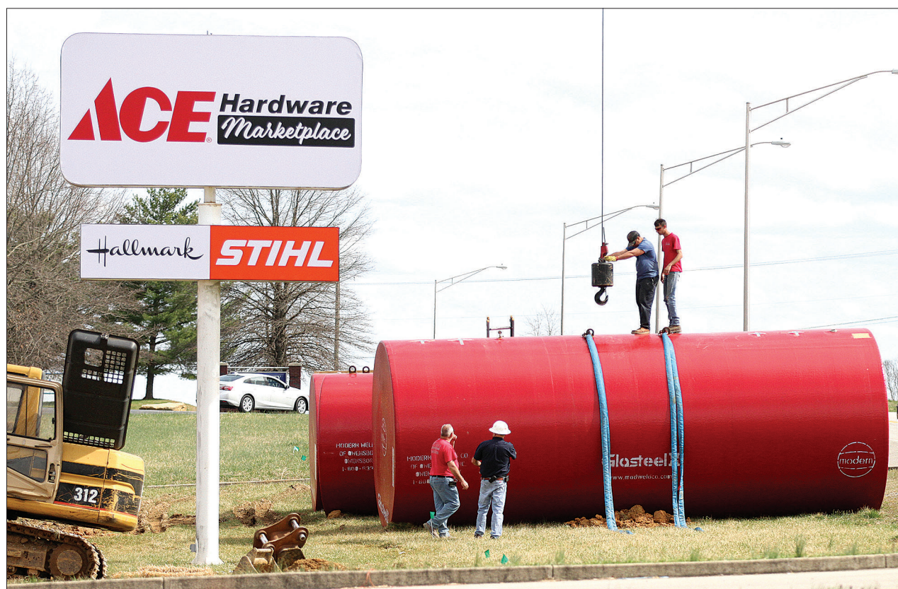
Tim Edwards Crane Co. put the gas tanks in the ground at the future My Town Country Store & Full Service Gas Station on Monday afternoon.
