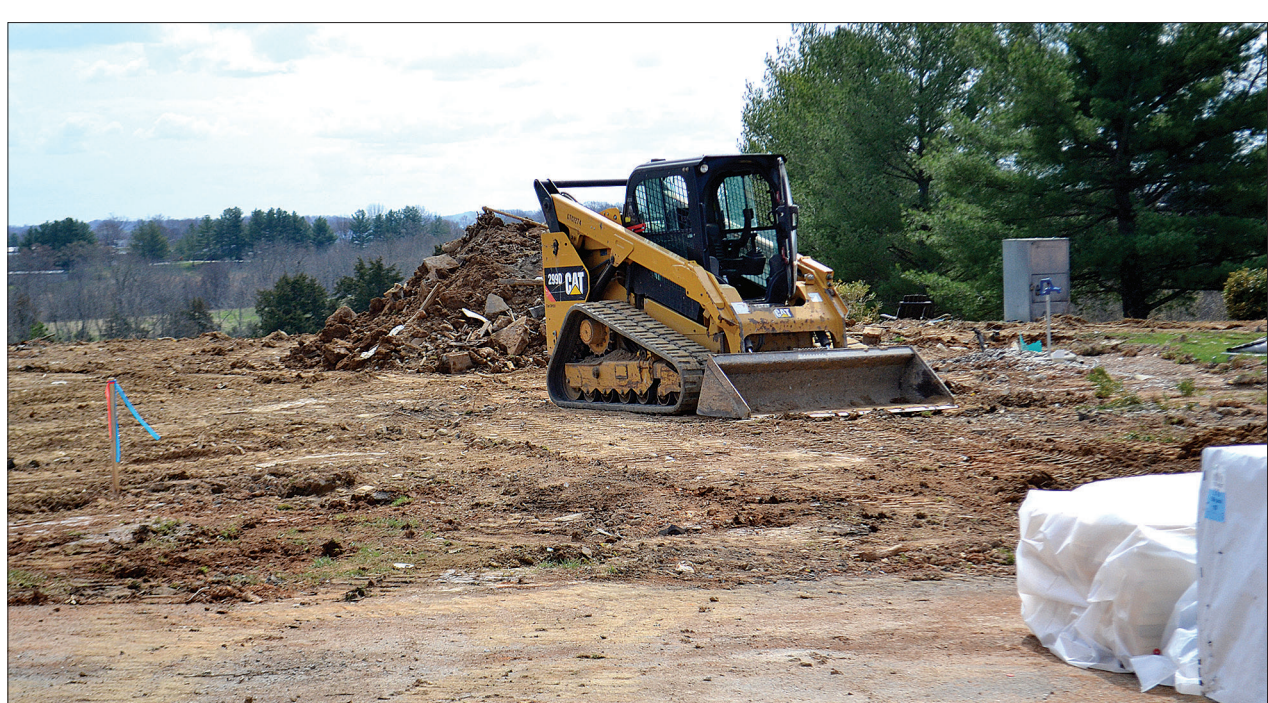
Work has begun on the new clubhouse at the Green County Country Club. While golf can still be played on the course, the clubhouse will allow for many more activities when completed.
