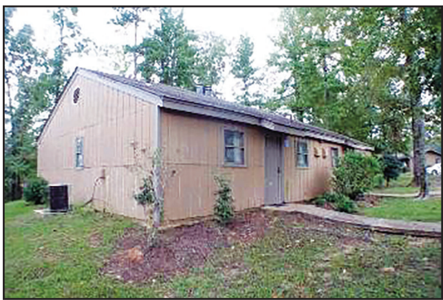
A cabin at Holmes County State Park, which is 'closed until further notice' for repairs, according to the state parks website. Mississippi's parks have suffered years of underfunding and lack of maintenance. (Mississippi Department of Wildlife Fisheries and Parks)
