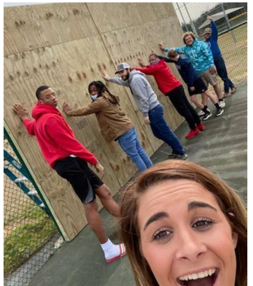
Students in Dwayne Connor's construction class built a wall that tennis players will use to practice their front and back swings. Setting it up on the courts were (back, l-r) Caleb Willis, Reggie Reid, Christian Mueller, Jusin Zellars, Caden Shaufelberger, Storm Bessinger, Jackson Bryant, (front, Brooks Lively. Tyler Coulson and Cody Doran are behind the wall fastening it to the fence.
