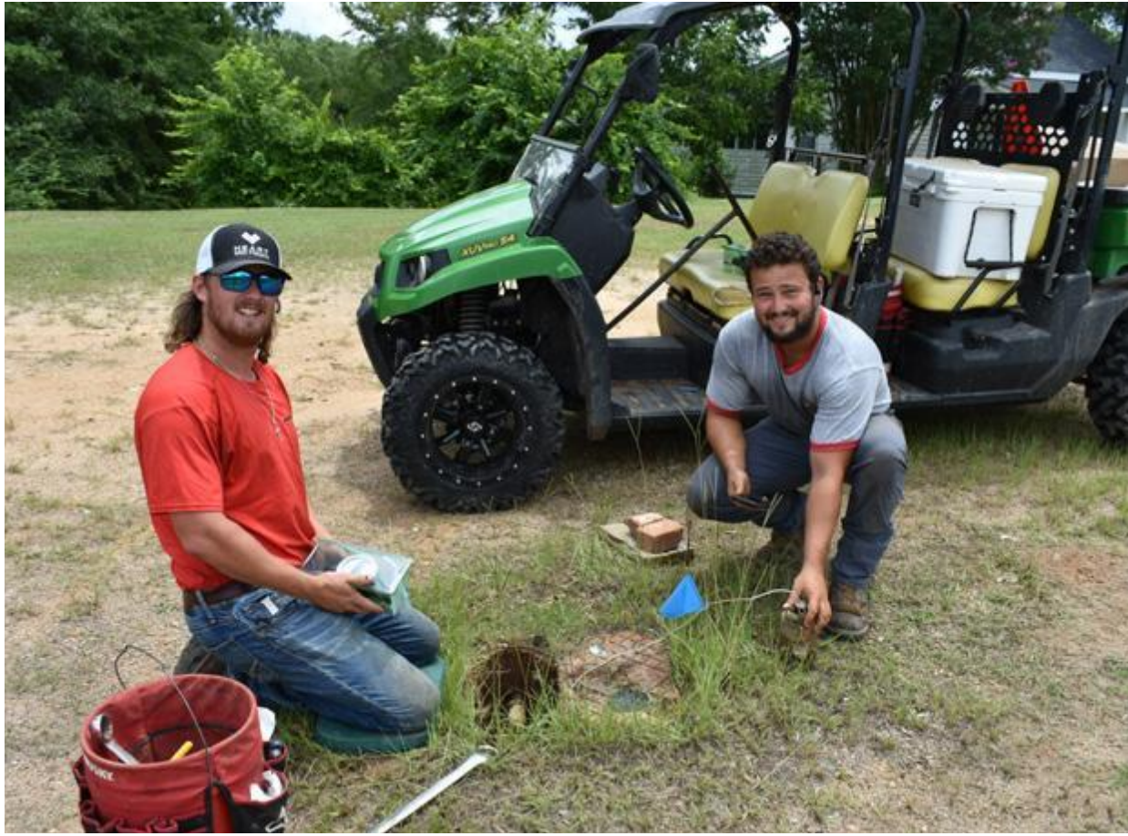
The Newton brothers Davis (left) and Charles with Brooks Brothers Construction were hard at work last week installing the new automatic meter reading system at a location on Washington Highway. The duo made short work of removing the old meter which Charles has his hand on.
