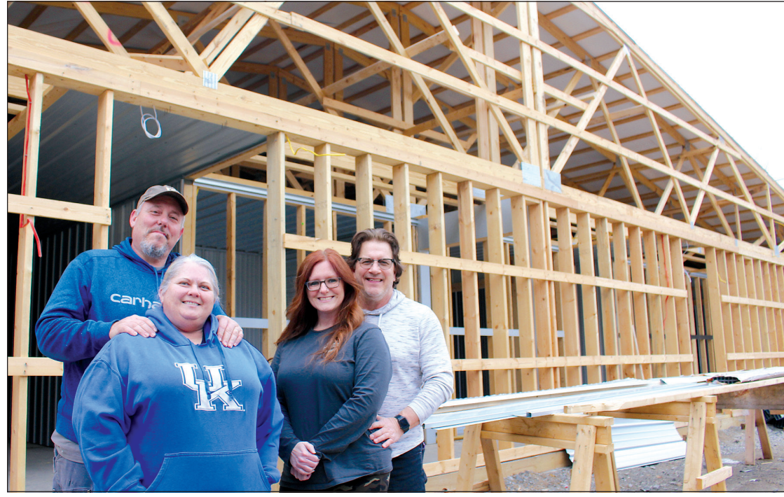
Lock-N-Stow owners, from left, Tom and Joyce Holt, and Stacy and Todd Wilson at their new facility in Russell Springs.
