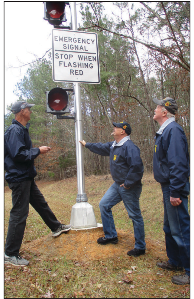
Inspecting one of the lights installed recently at the Sandy Branch Volunteer Fire Department are (l-r) firefighters Glenn Heffner, Sean Boyce and Ralph Layton.
