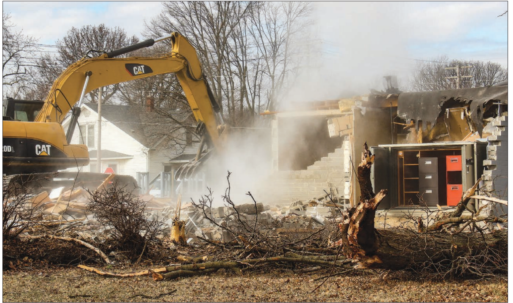
AN EXCAVATOR TAKES a bite out of this building at 600 E. Southline Rd. (U.S. 36). It housed an office for former mayor Chris Hill for many years. According to Douglas County tax records, the building was sold in 2017 to Sarus Developers LLC in Champaign for $375,000. Photo by David Porter.
