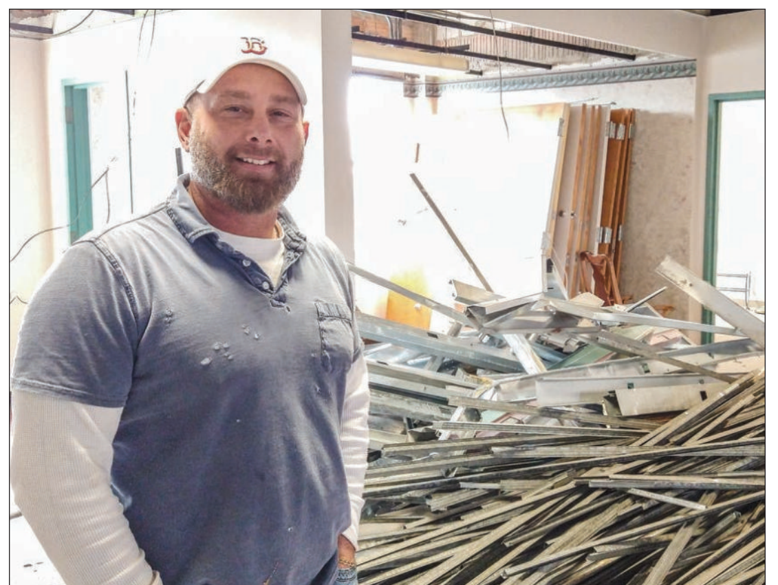
CHRIS ROBINSON stands in front of a pile of debris — old drop ceiling rods — at the former Jarman Hospital. He purchased the building earlier this month and is renovating it for apartment units. The outdated drop ceilings will be drywalled, he said, and the first floor carpets and tile in the foyer will be replaced with marble-like tiles. Photo by David Porter.
