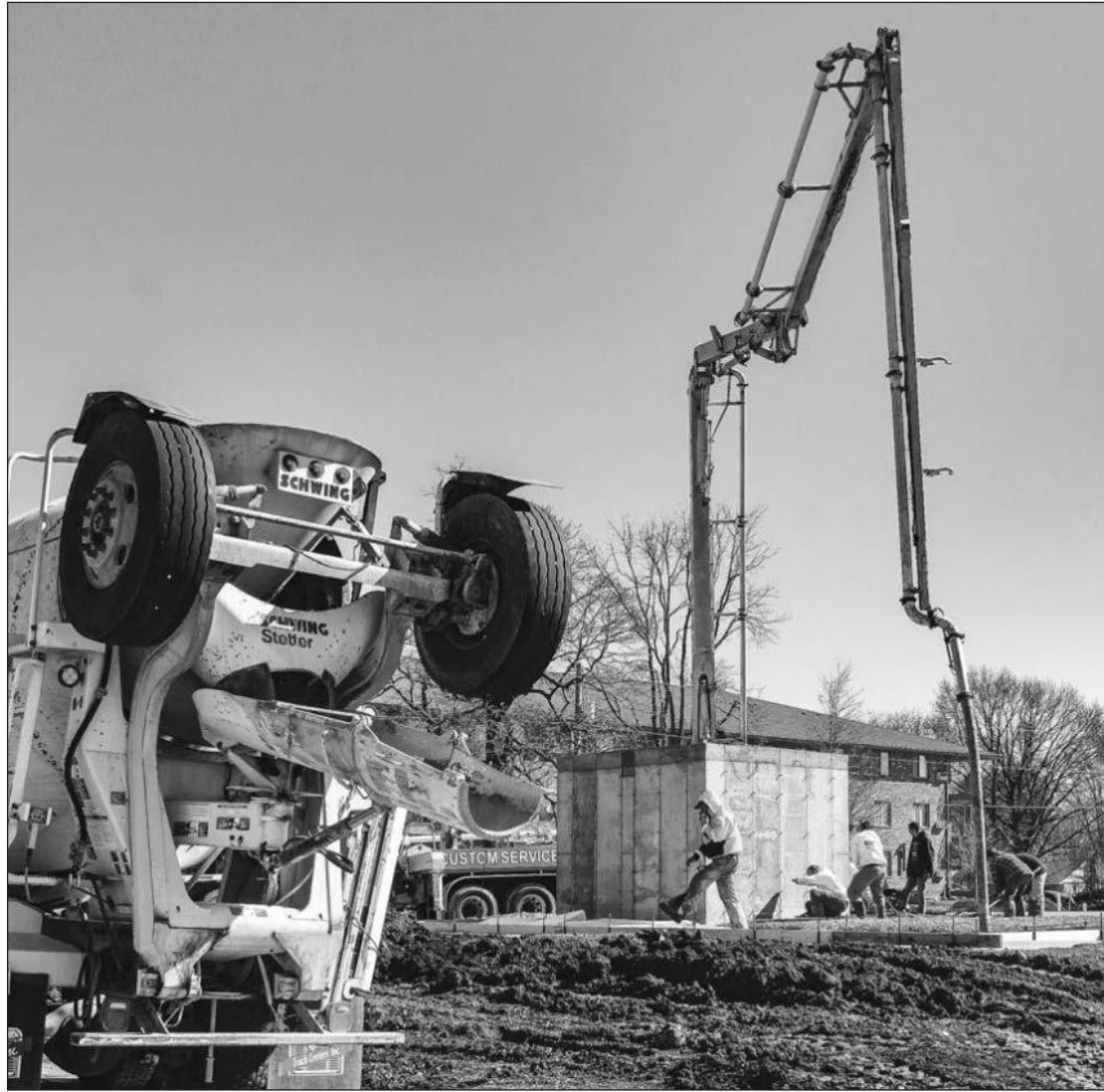
JODI'S ASPHALT IN DANVILLE pours concrete for the new Longview Bank on Rt. 36 in Tuscola. Jodi's is owned by Jodi and Rob Gentry. Rob, kneeling, is a Tuscola High School graduate. Photo by David Porter.
