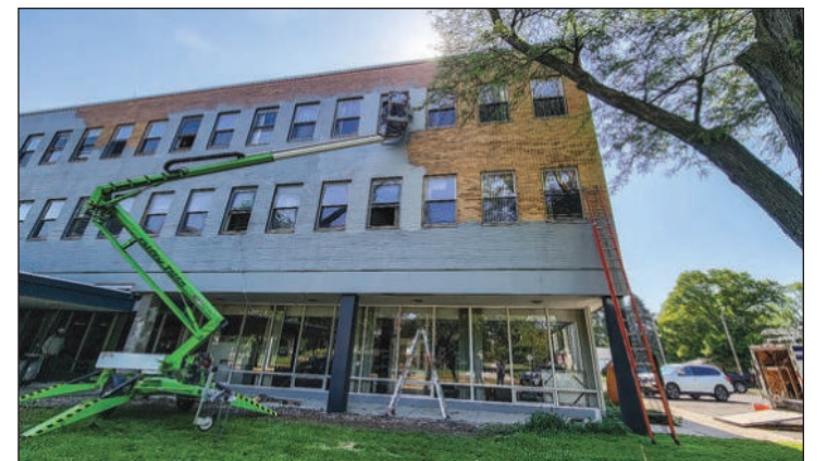
THE FORMER JARMAN HOSPITAL in Tuscola, now being turned into apartments by Chris Robinson, is getting an updated look. Aaron Weaver is painting the building gray. Photo by Jennie Porter.
