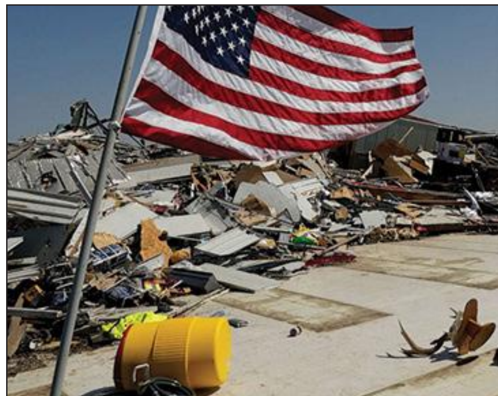
An American flag files on the slab of a tornado destroyed hardware store in Rolling Fork, Miss., Mar. 25, 2023.
