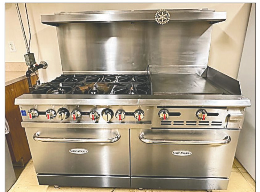
A NEW SIX-BURNER stove has been installed at the Community Center following fundraising by the Arcola Rotary Club. Submitted photo.
