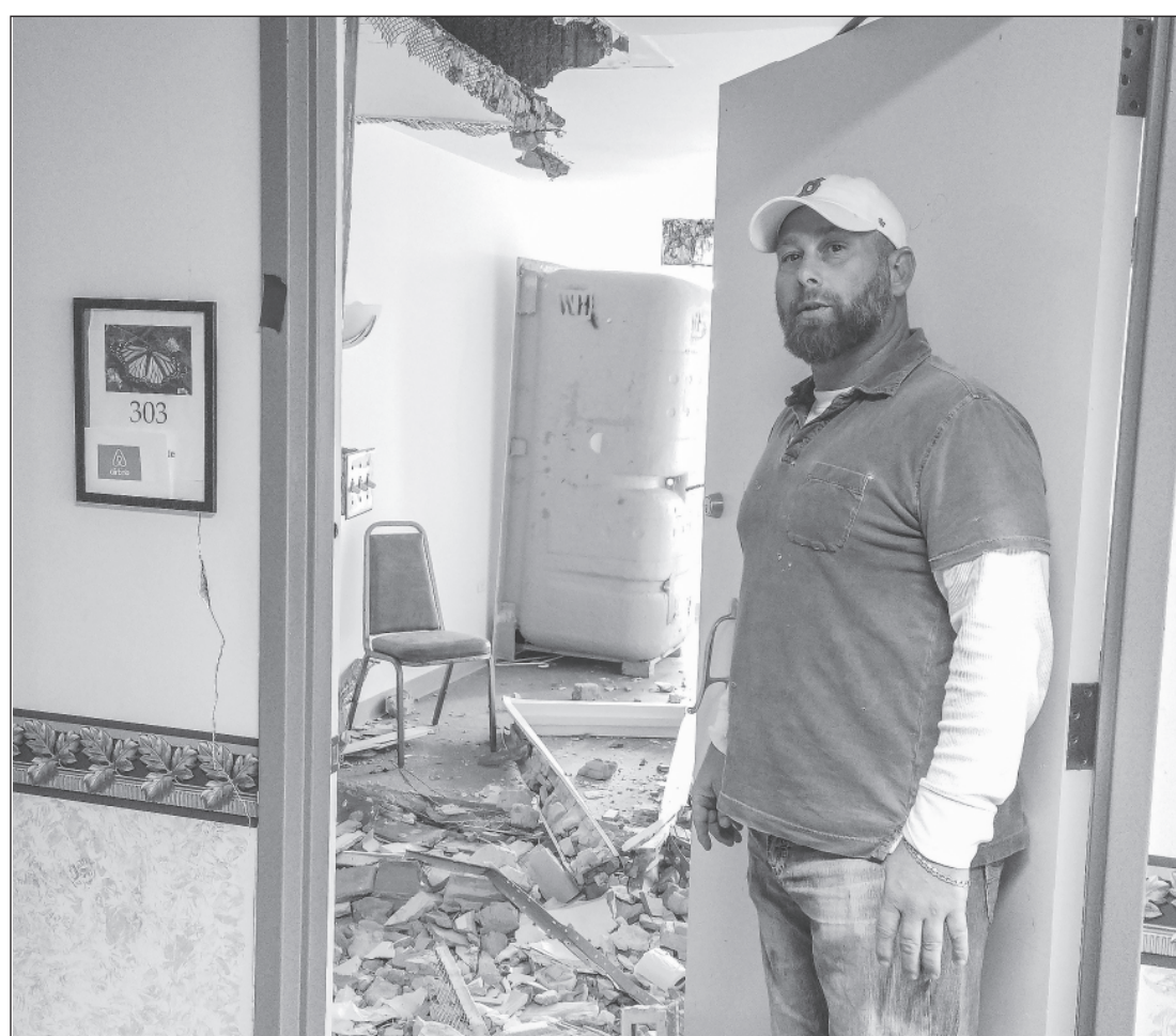
CHRIS ROBINSON, current owner of the old Jarman Hospital, shows demolition work in an upstairs room last year.
