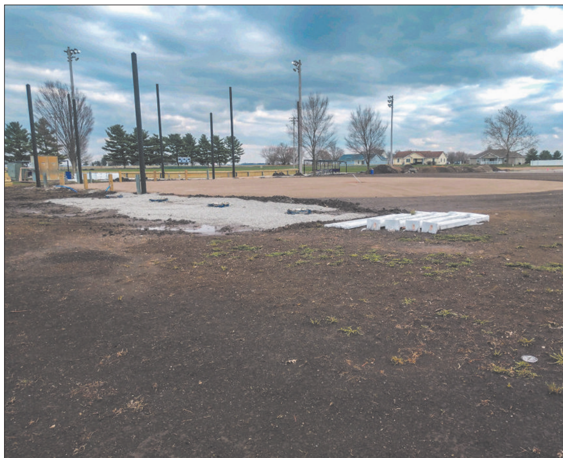
A NEW FIELD to be used for t-ball and coach-pitch is taking shape at Arcola's Moore Memorial Park. The high school baseball field is in the background.
