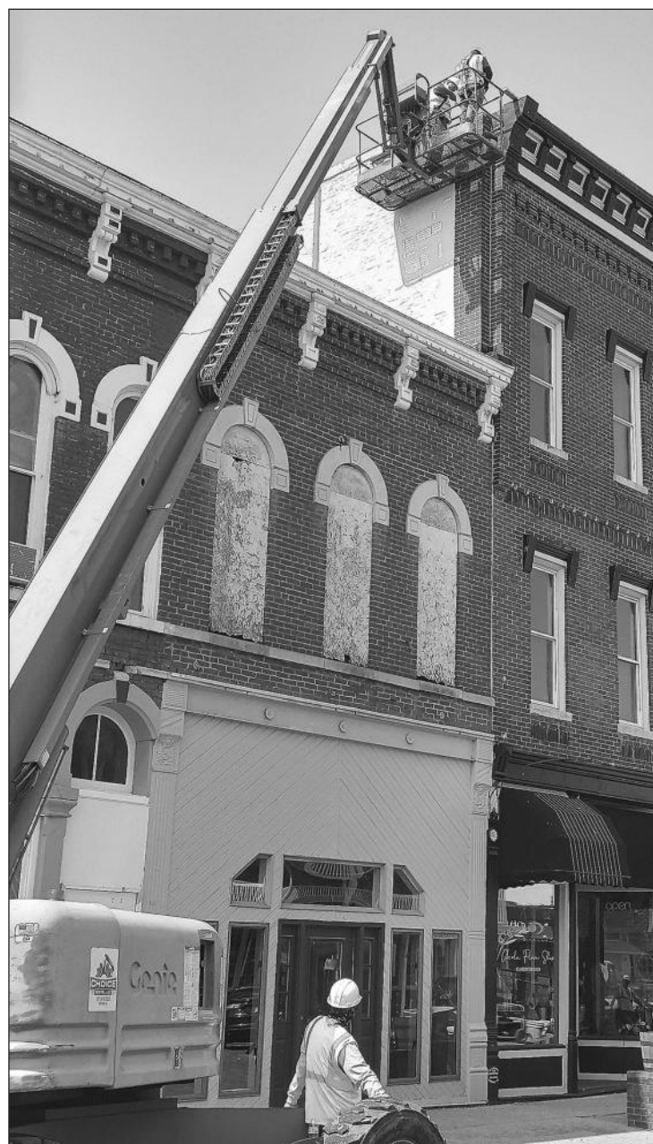
WORKERS USED a lift last week to repair a hole in the roof of one of Arcola's historic downtown buildings. The city pitched in to help cover the costs of the repairs. Photo by David Porter.
