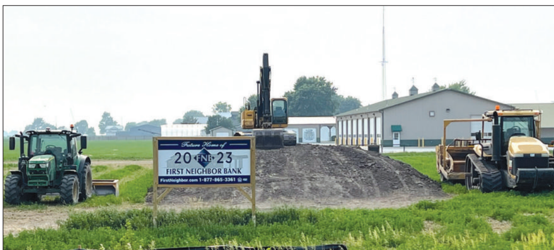
First Neighbor Bank broke ground on May 30, 2023 at the site of its new Arthur, IL location (601 S Vine St) at the intersection of 133 and Vine Street. Construction of the facility will follow on the new Arthur banking facility and First Neighbor anticipates that it will open in the first quarter 2024.
