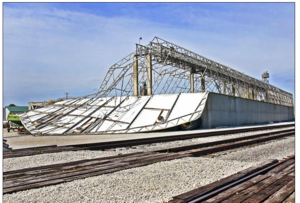
THE EQUITY in Galton suffered heavy damage in Thursday's storm, which brought 80 MPH hurricane-level winds. Some parts of the county also saw fist-sized hail. Trees and power lines were downed in Arcola, Tuscola and Villa Grove leaving some residents without power for days. Semis were overturned on I-57. The storm followed several days of unhealthy haze caused by wildfires in Canada. Photos by Nancy Rairden.
