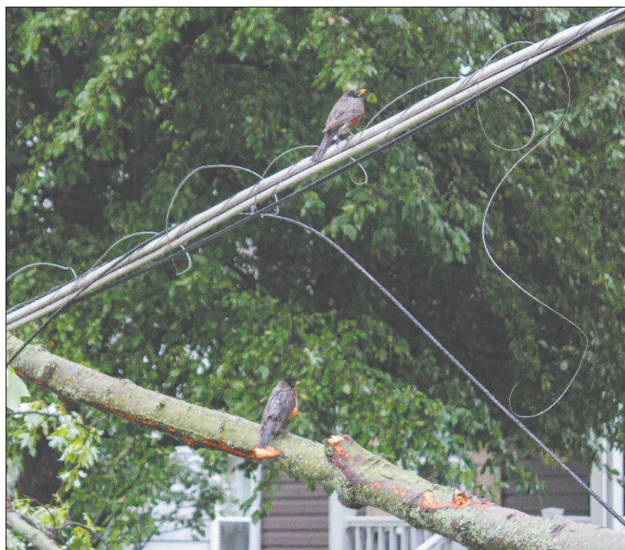
A PAIR OF ROBINS seem unfazed by downed power lines and limbs as they roost among the chaos Thursday in Tuscola. Following days of unhealthy air caused by Canadian wildfire smoke, a storm brought hurricane-level winds and large hail to parts of the county causing substantial damage to trees, homes and businesses. Photo by David Porter.
