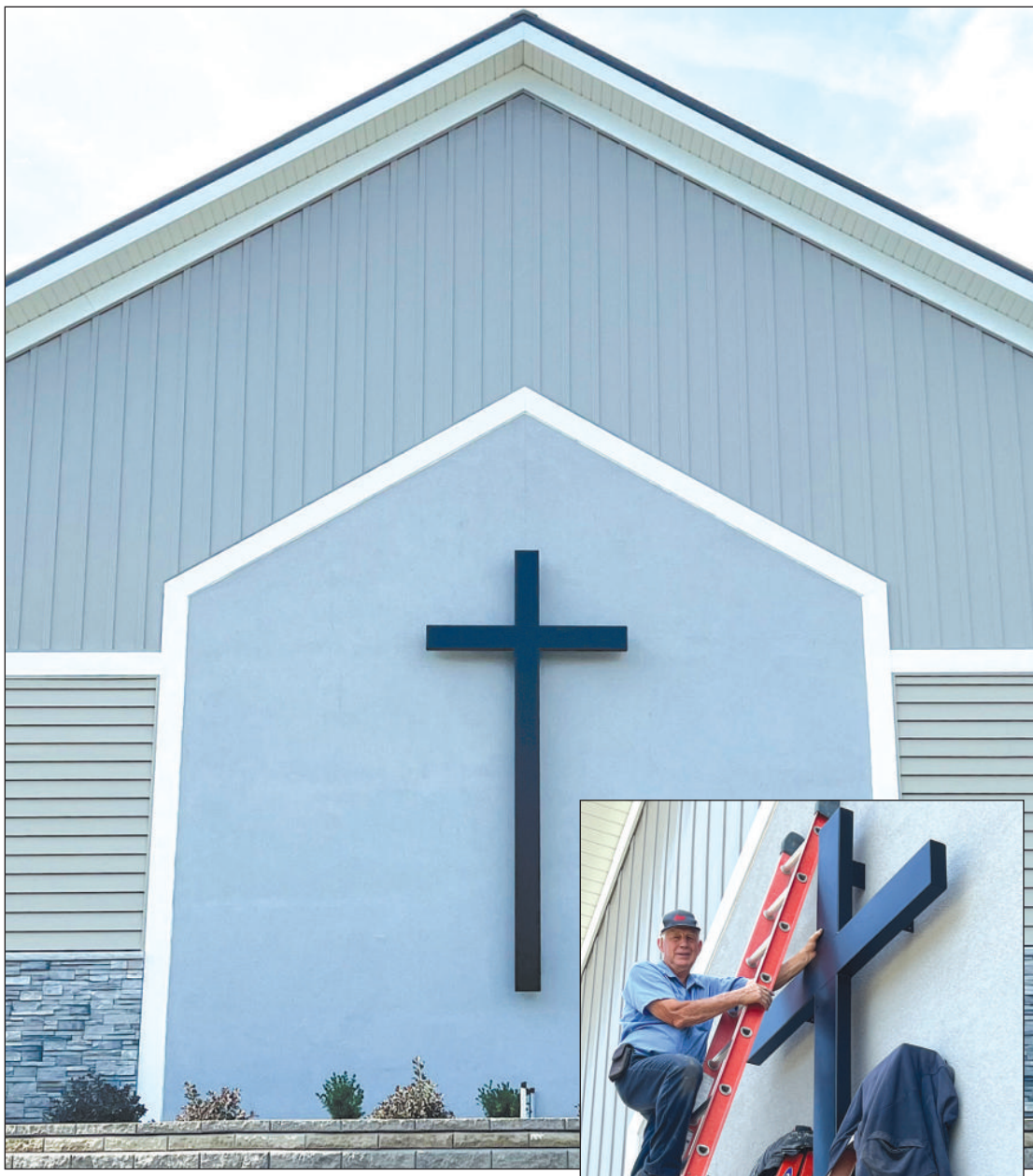
THE FINAL TOUCH. Almost 28 months to the day, the new cross was placed at the Sunnyside Mennonite Church following the fire that totally destroyed the church back on March 26, 2021. The original cross, made of fiberglass, was partially destroyed in the fire and thought to be salvageable however that was not the case. The new cross constructed of aluminum was made locally by Frontier Manufacturing, LLC just outside of Chesterville. Loyd Gingerich on the ladder had help from Richard Beachy and Noah Yoder two other members of the building committee (not pictured) on the project. The church is hosting an Appreciation/Celebration on Saturday, August 12 that includes a tour of the new facility, food, and ending with worship.
