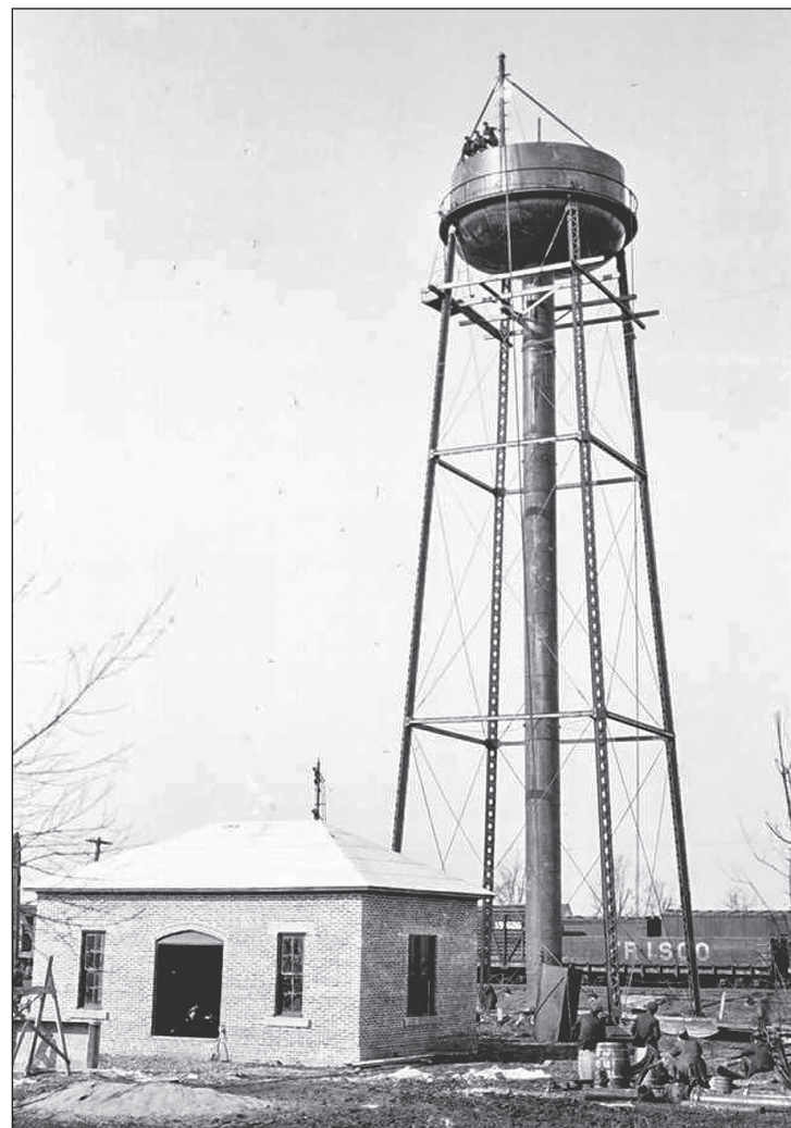
WATER TOWER under construction, 1914, at 314 W. Progress St. In 1911, the Village residents voted 125-95 to erect a 100-foot steel tower holding 50,000 gallons of water and install a water system for $9,500. Previous to this time, each house and most businesses had a private well.
