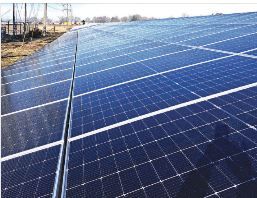
WESTWARD VIEW of Gail Technology solar array. Photo by Tony Hooker.
