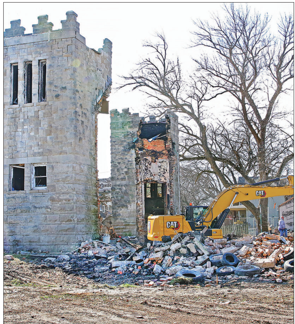
BEFORE IT WAS KNOWN as the "Castle Mall," the structure was a former Presbyterian church. Photo by Nancy Rairden.
