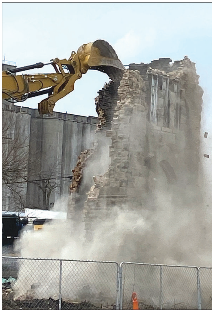
HEAVY MACHINERY from Ezccll Excavation tears down part of the burnt-down "Castle Mall" structure. The building burnt down on July 9 in a suspected arson case. Photo by Michael Carroll.
