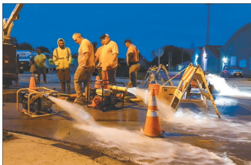
THE CITY HOOKED UP A THIRD PUMP to try to remove water from a pit at Main and South Central. Foreman Denny Cruzan said the repair would take only about 15 minutes if they can clear enough water out. Photo by David Porter.
