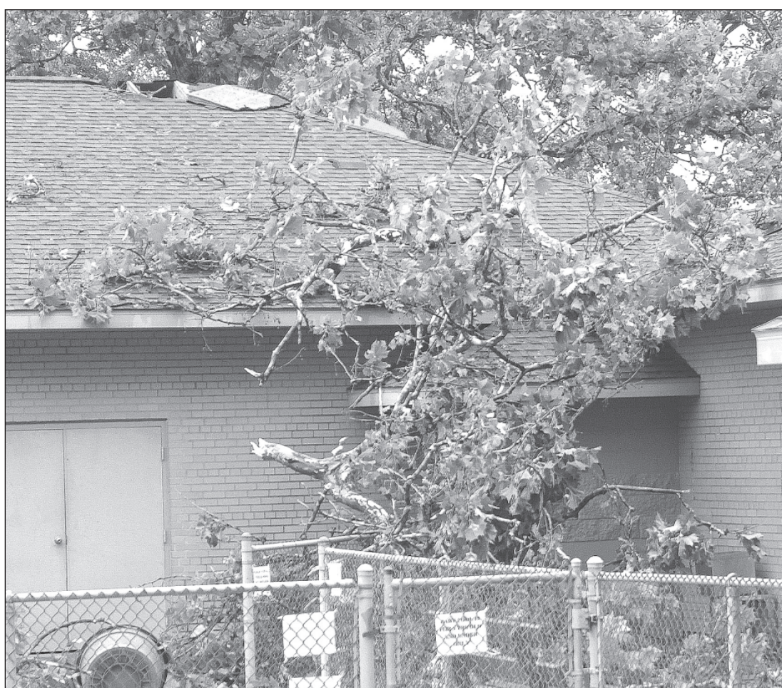
A FALLEN TREE IN ERVIN PARK punched a hole through the roof of the Tuscola pool building. The city will make a determination on June 3 when to open the park and the pool. Photo by David Porter.
