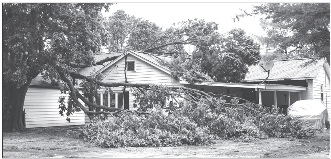
BRANCHES FROM TREES damaged roofs around Tuscola. Crew workers worked throughout the weekend to clear the roads and then roofs of debris. Photo by David Porter.
