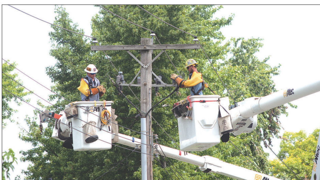
AMEREN WORKERS perform maintenance on a powerline located on North Parke Street. Workers performed maintenance while a customer requested a power shutoff. Photo by Dominik Stallings.
