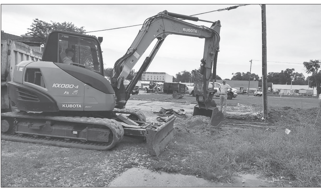
BILL WILSON EXCAVATES GRASS AND DIRT in the alley between North Central Avenue and East Sale Street in Tuscola. The alley and greenspace are being redone as part of Phase 2 of the Downtown Alley Improvement project. Photo by Jaclyn Henry.
