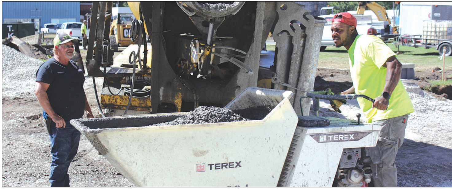
TYRONE JASPER, right, delivers a load of cement to workers smoothing out concrete in the alley between North Central Avenue East and East Sale Street. The alley is being remade as part of the Tuscola Downtown Improvement project. Photo by Dominik Stallings.
