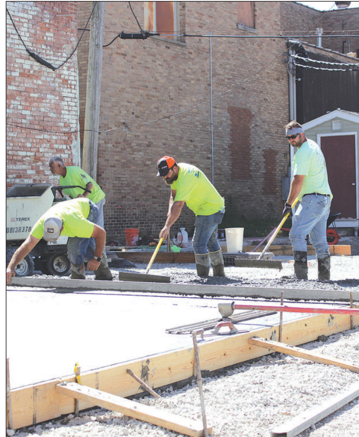
JARED QUIK, Tim Zerussen and Jeremy Creech smooth out freshly poured concrete in the alley between North Central Avenue East and East Sale Street. The green space next to the Tuscola Community Building will be worked on next. Photo by Dominik Stallings.
