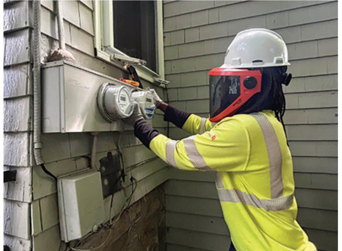
Eli Jones, an electric meter technician for Grid One Solutions, a subcontractor for Rhode Island Energy, installs two smart meters on a house in Newport on Friday, Sept. 12, 2025. Pending federal approval, South Carolina plans to roll out its own energy-saving program for homeowners. (Photo by Janine L. Weisman/Rhode Island Current)
