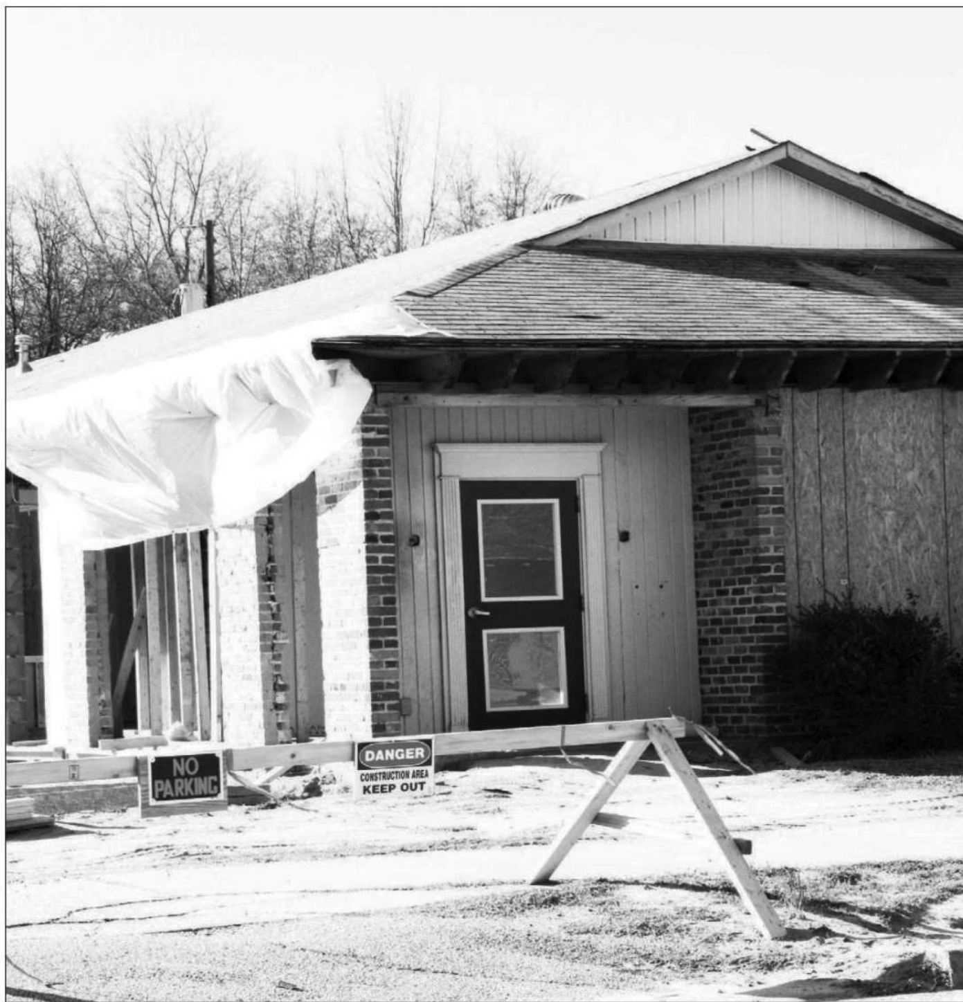
Work has begun on renovating and expanding the old Kershaw Community Health Care building on East Marion St. into a new CareNet Clinic to provide health care for the community's uninsured and underinsured residents. Photo by Billie Deaton.
