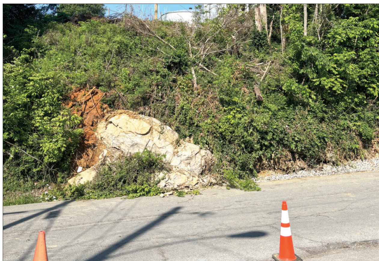
West Hodgenville Avenue from Second Street to Hidden Valley Road is closed. The small hillside near the water tower has fallen very near to the edge of the road making any traffic a potentially dangerous situation. Residents of Graham Court and Lewis Court, two of the nearby neighborhoods, have been forced to use the lower entrance to their homes and cannot access their homes coming from the area near Adanta and the Cumberland Presbyterian Church.
