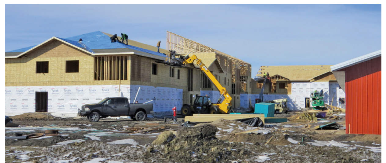
With the spring weather warming, activity on the new 35-unit apartment complex in Barnesville is picking up speed. The building is being wrapped with Tyvek. Roofers are nailing down buffalo board to the rafters. Windows are being installed. It's a busy scene but still a long ways from being done. Look for a fall opening of the apartments.
