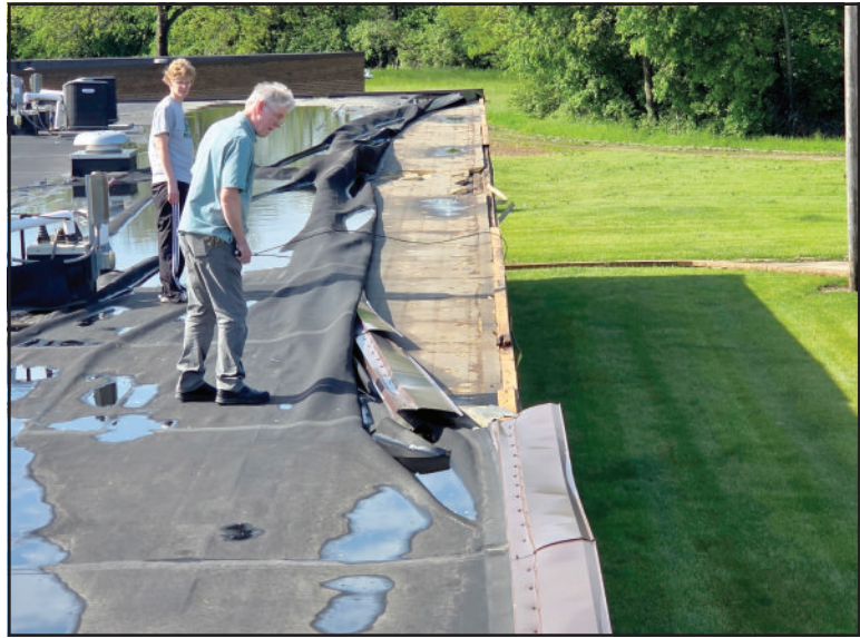
Damage to the Midland Middle School roof in Sparland.
