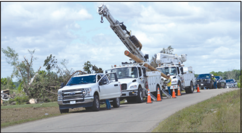
Numerous Ameren trucks on the scene working to restore power
