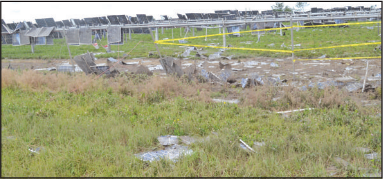
After passing north of Washburn, the tornado struck a wind farm doing major damage and spreading debris around the area.
