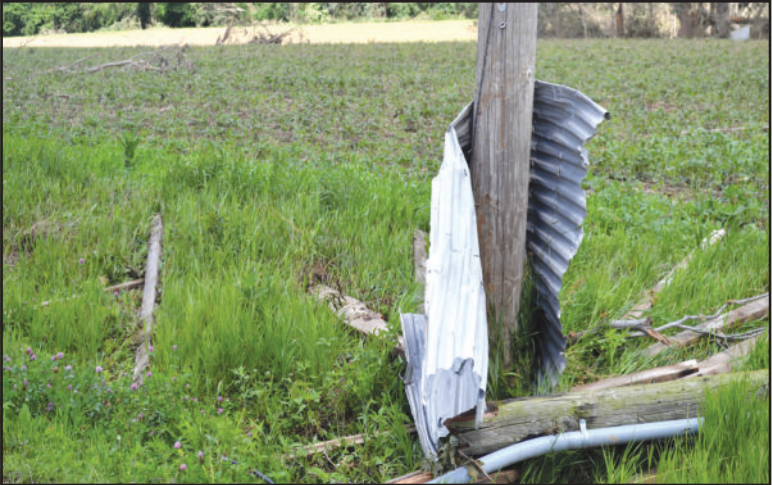
Metal wrapped around a utility pole speaks to the volume of the wind.
